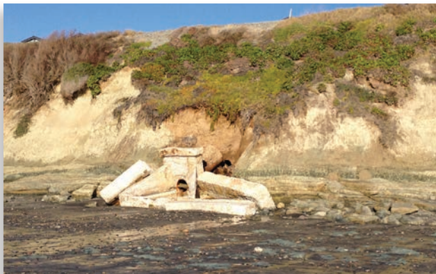
Br 244.3 drainage outlet to be stabilized
