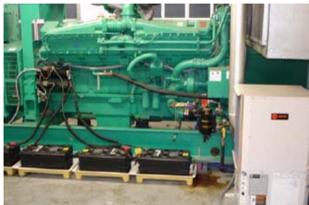
Figure 9 Example of Heat Pump (On Right) For Back-Up Generator
