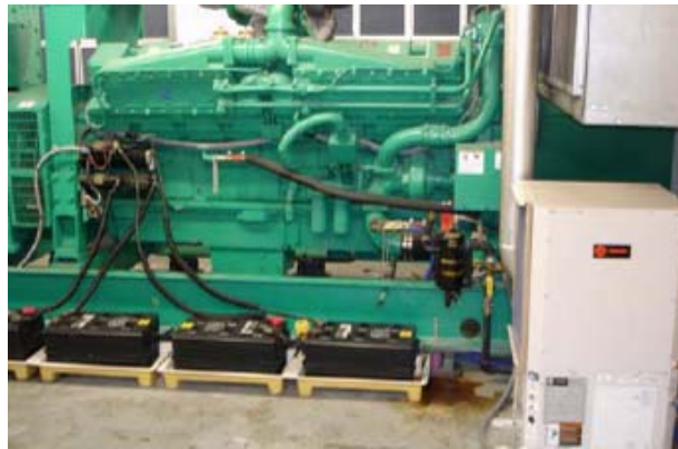
Figure 35 Example of Heat Pump (On Right) For Back-Up Generator
