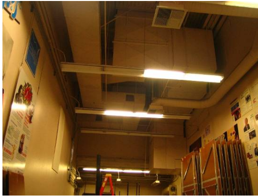
Figure 29 Lights at Back Stage/ Loading Dock
