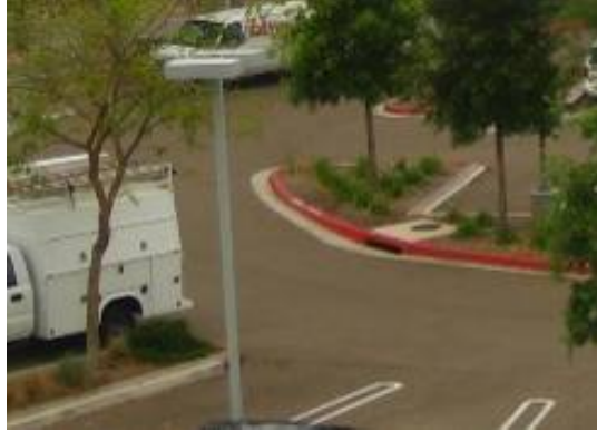
Figure 7 Pole Lamps in Parking Lot
