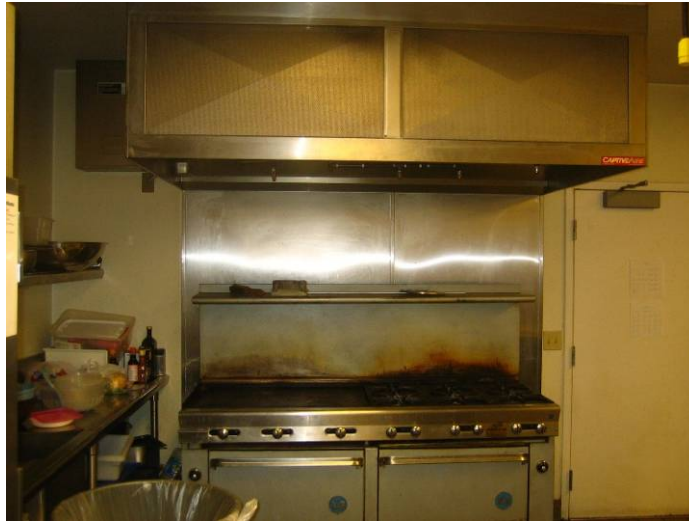
Figure 23 Existing Kitchen Hood
