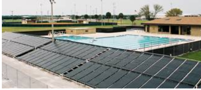
Figure 12 Example of Commercial Pool SWH installation
