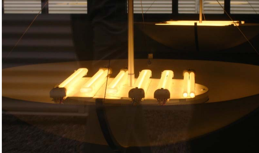
Figure 4 Main Lobby Fixtures with Biax Lamps
