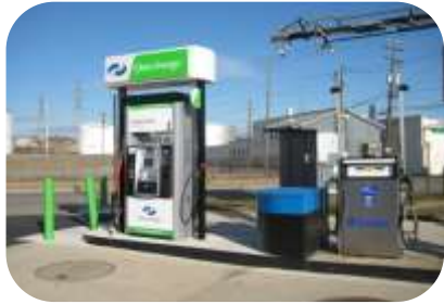
Two new CNG stations (EDCO) added
