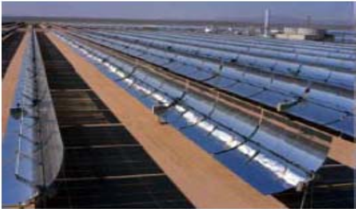
Central – Kramer Junction (CA) Solar Electric Generating Station
