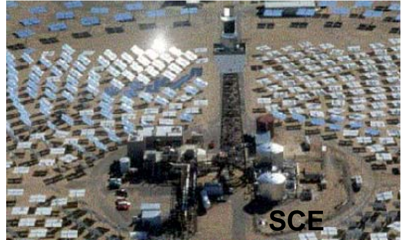
Solar Two Central Receiver (Power Tower)
