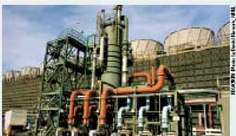
Cooling towers and piping at a power plant at The Geysers.
