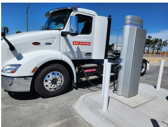
Figure 5. A DC fast charger installed by SDG&E at Truck Net, north of the Otay Mesa Port of Entry in California. Photo: SDG&E
