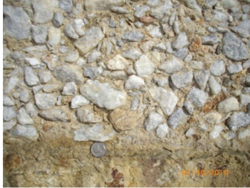
Figure 6 - 100-year-old railway culvert outfall built in 1910 on the beach in Del Mar at MP244.3
