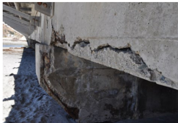
Figure 1: Chloride Induced Corrosion
