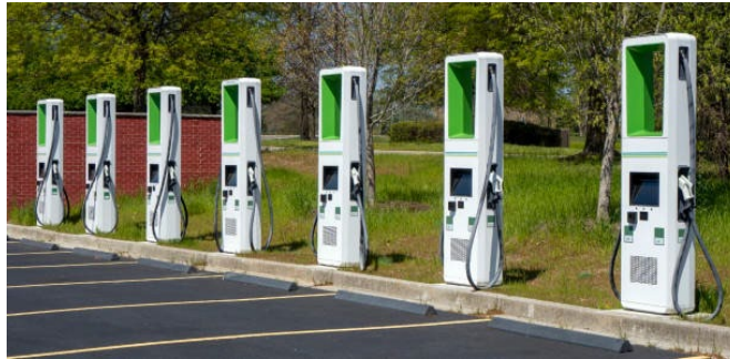
EV charging stations, Source: iStock
