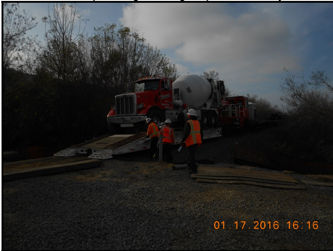
Bridge 247.7 – Concrete for the two interior bridge's CISS piles is being trucked in via TowRailer cars during train free periods (AWWs). The trucks are being loaded onto the TowRailers at Bridge 247.7 and are then pulled by the Shuttlewagon to the two interior bridges (See below photo).
