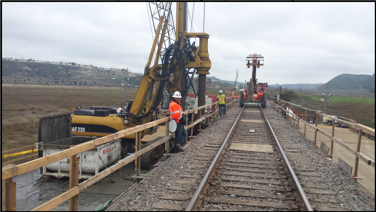
Bridge 246.9 – Exterior CISS piles for Bridge 246.9 continue to be installed during the day under Form B protection.
