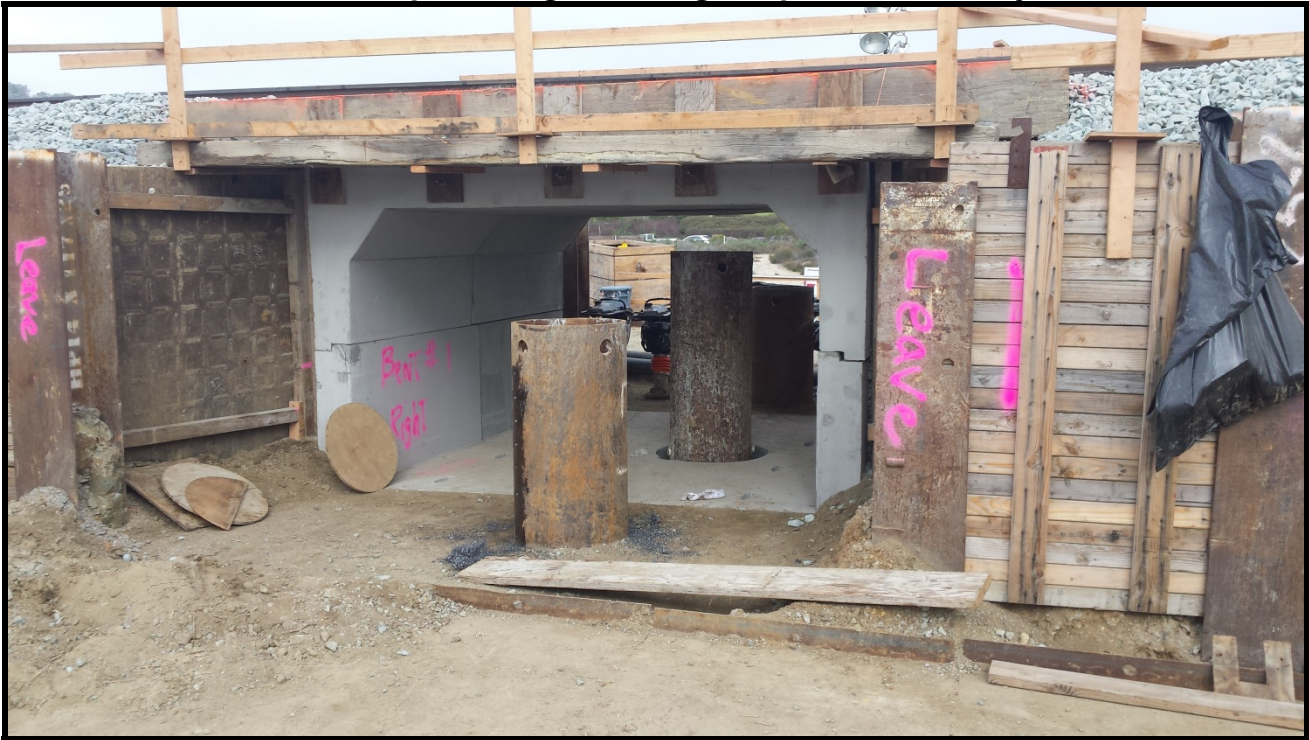
Bridge 246.1 – The two Jump Spans at Abutments 1 and 11 were installed during the Jan 16-17 AWW
