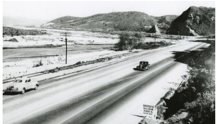
Camp Pendleton construction of Vandegriff Rd (circa 1940s). Photo by Official USMC.
